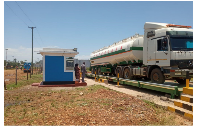
● The East Africa Petroleum Transports Association (EAPTA) constructed a new Self-Regulating Weighbridge opposite Kenya Pipeline Company Depot, Kisumu, to enhance Axle Load Compliance.
